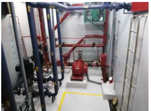
Firefighting and Water Distribution Equipment
