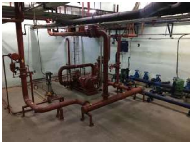
Firefighting and Water Distribution Equipment
