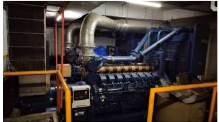
Standby Power Generators
