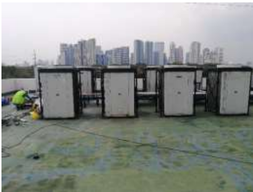
Air Conditioning Units
