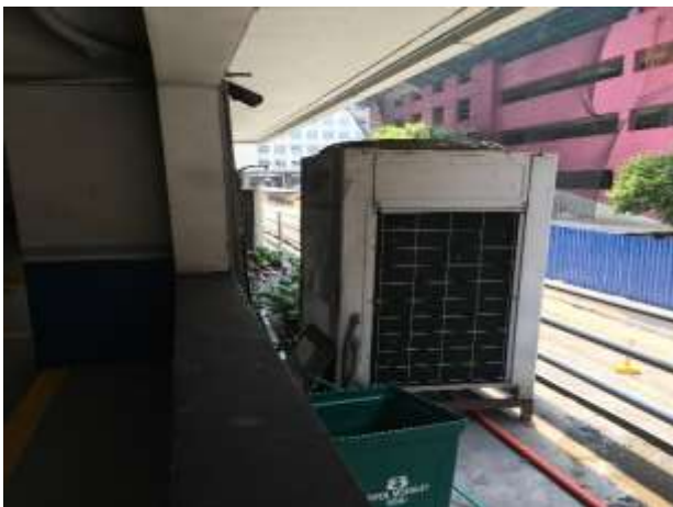
Air Conditioning Units
