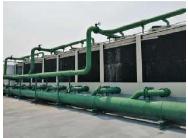
Air Conditioning Units
