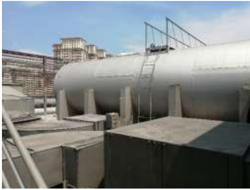
Overhead Water Tanks
