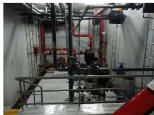
Firefighting and Water Distribution Equipment
