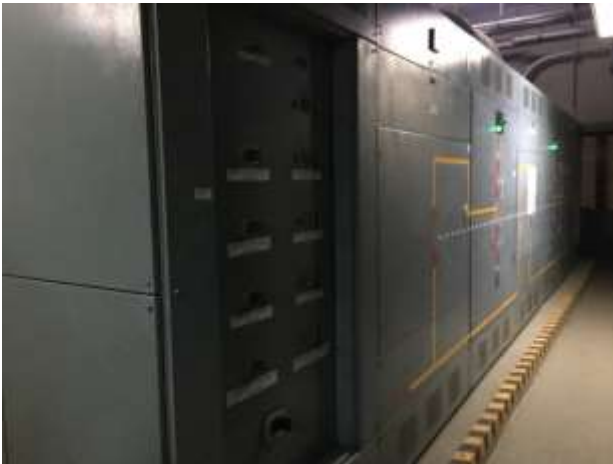
Electrical Distribution System
